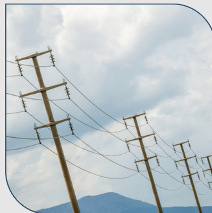
Power Distribution Line Insulators
